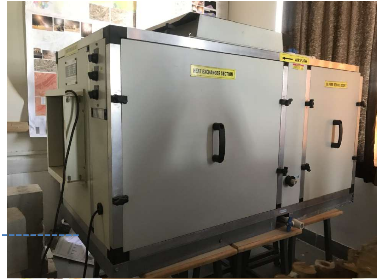
Radiant Cooling System
