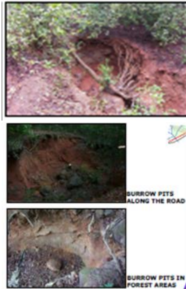
Figure 2: Burrow pits along the road and in the forest area - occurs due to natural settlement of soil in particular area
