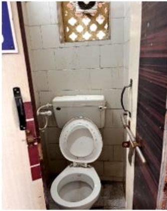
Figure 12. toilet for the disabled
