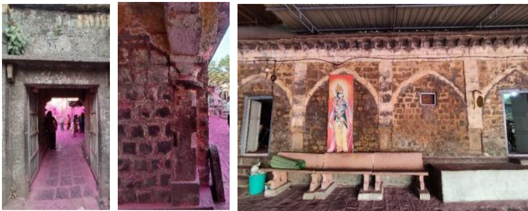
Figure 08: The present state of the temple structure; temporarily repaired with random plastering etc.
