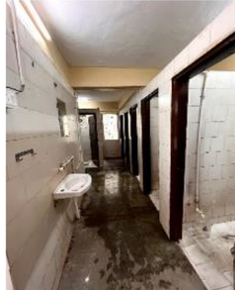
Figure 13. less ventilation and light
