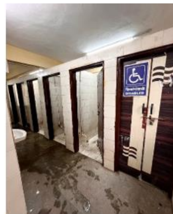
Figure 16. LOCKED PWD WASHROOMS
